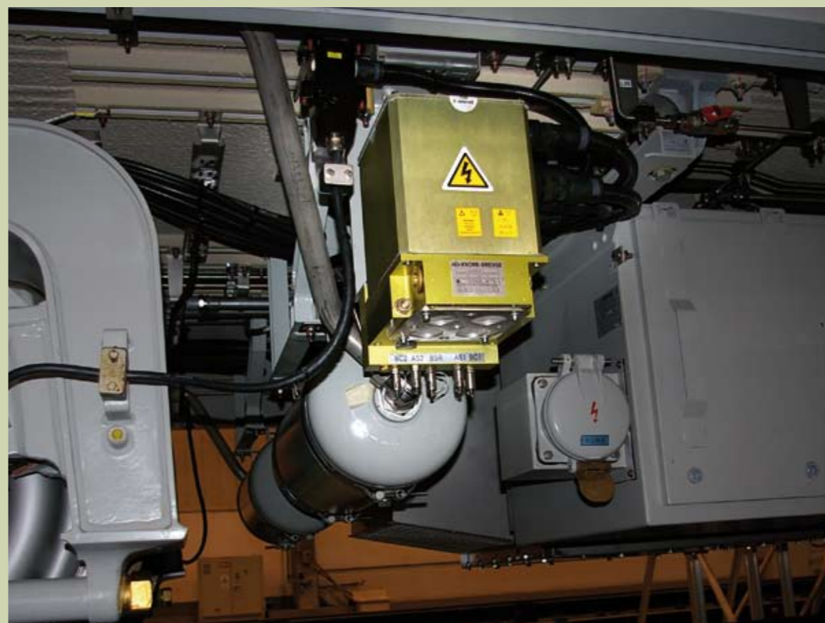
Traditional mounting of a EP2002 control valve in front of a horizontal reservoir EP2002 Cube can be installed in the same space.
